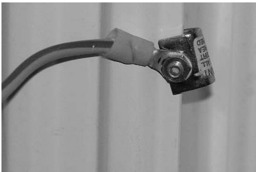
Fig. 13.10 Earthing clip on radiator.
