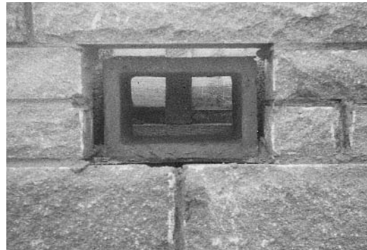
Fig. I.13 A similar liner built into a cavity wall in the wrong place.
