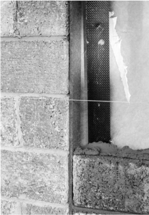
Fig. 3.37 Faulty joint being built in the block cladding of a timber frame house.
