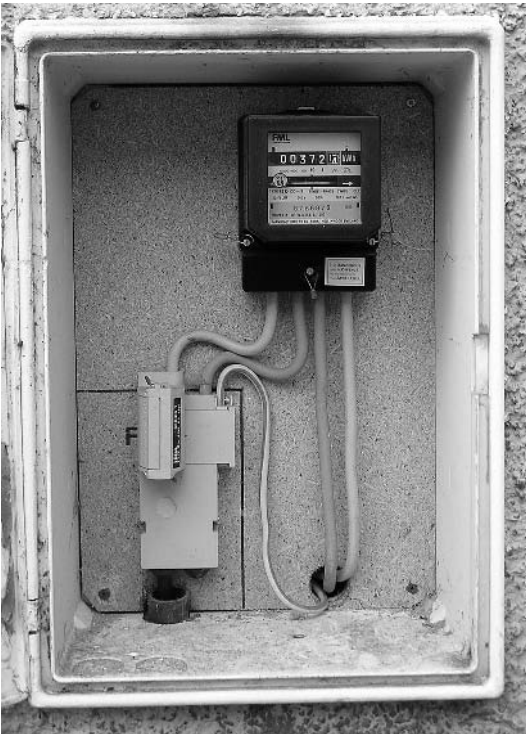
Fig. 13.2 Single phase cut-out and meter in cupboard.
