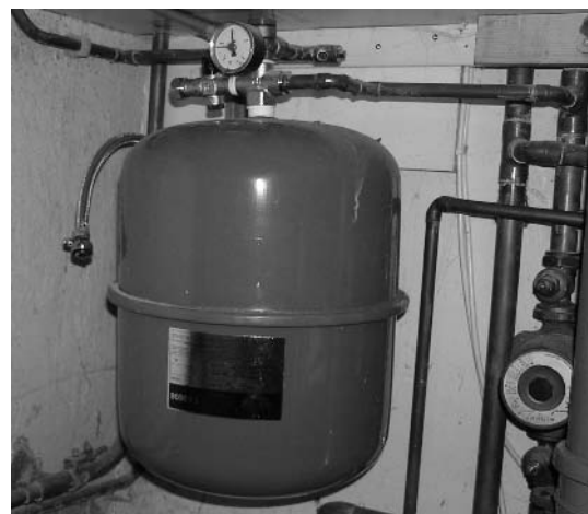
Fig. 12.33 The pressure vessel and valve arrangements of a pressurised central heating system.
