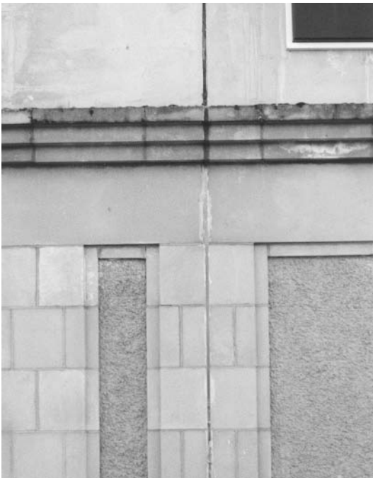
Fig. 3.36 A mastic sealed joint in a complex wall of reconstructed stone and rendered blockwork.
